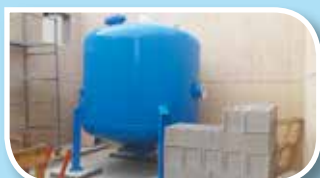
(a) cuve filtration
